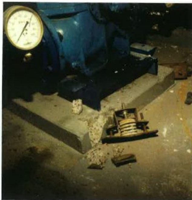
Figure 14 The proper housekeeping pad footprint is important to ensure the proper distance from the anchor bolt to the edge of the pad. A wider pad would have prevented this failure.
