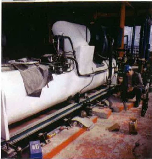
Figure 13 The Northridge quake lifted this chiller and housekeeping pad off the ground and slammed it into the structure.
